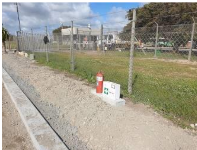
Image 1: Fire extinguisher on site.
